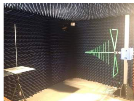
1 of 3 EMC Test Chambers
